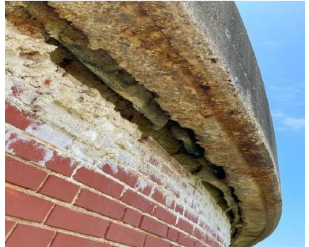
Digester No.2 Corrosion and Potential Sulfur Deposits
