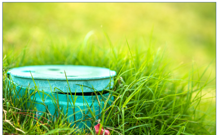
► Uncapped lateral cleanout pipes
