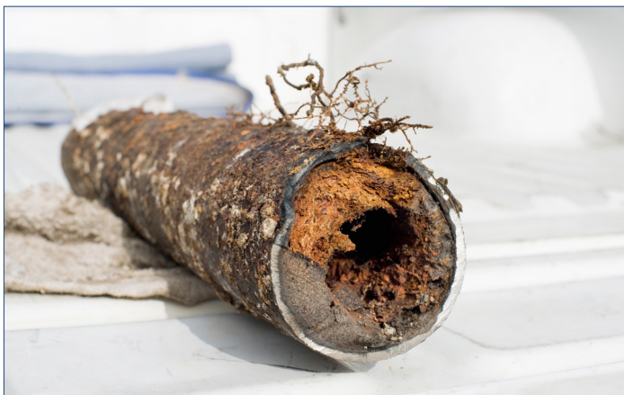
► Blockages or clogs in the pipes
