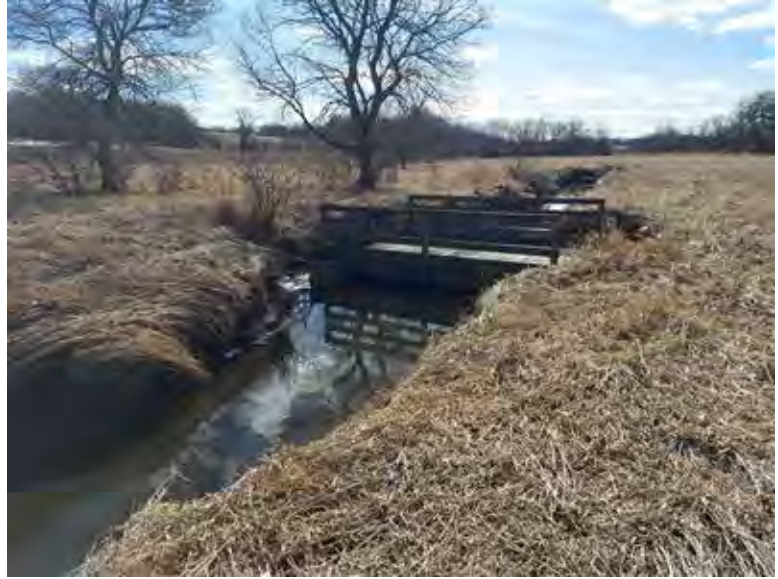
March 7, 2023: Bridge sitting on the bottom of stream, downstream of aerator
