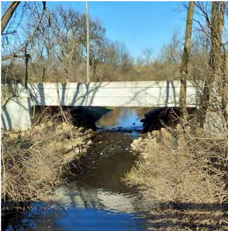
Figure 11 - BMC at Old PB on April 21, 2022 – USGS Gage flow and Photo, normal the District’s operation
