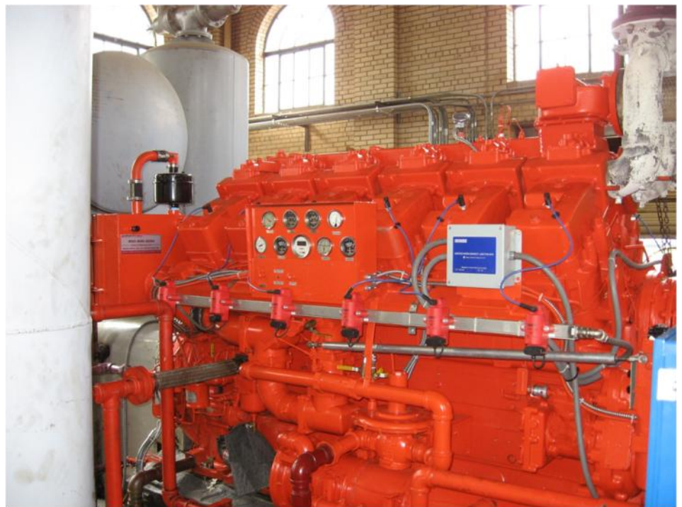
Rebuilt East Blower Engine installed in the East Blower Building
